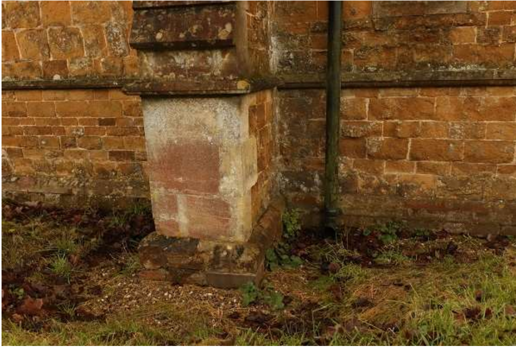
Figure 19 – Vegetation growth in frenchdrain at rear of church
