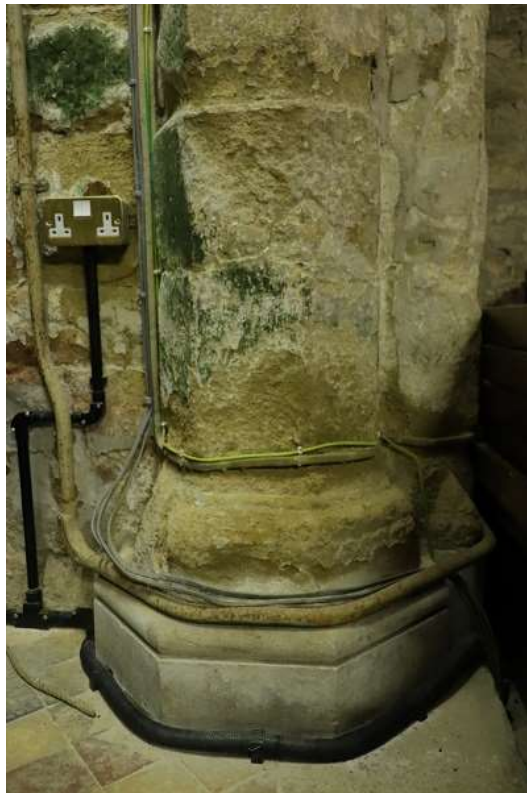
Figure 24 – Tidemarks and spalling of west pillar
