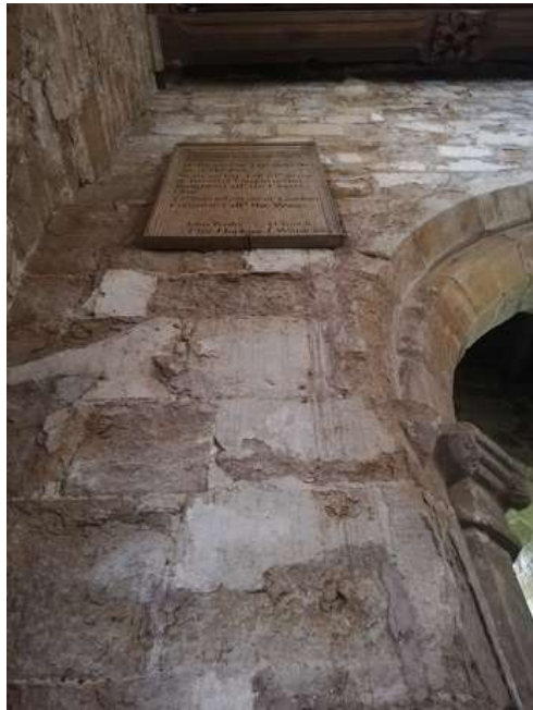
Figure 13 – Drip marks on west wall
