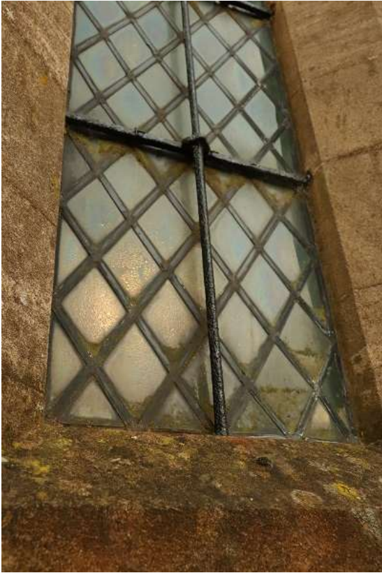
Figure 31 – Encrustations on window exterior
