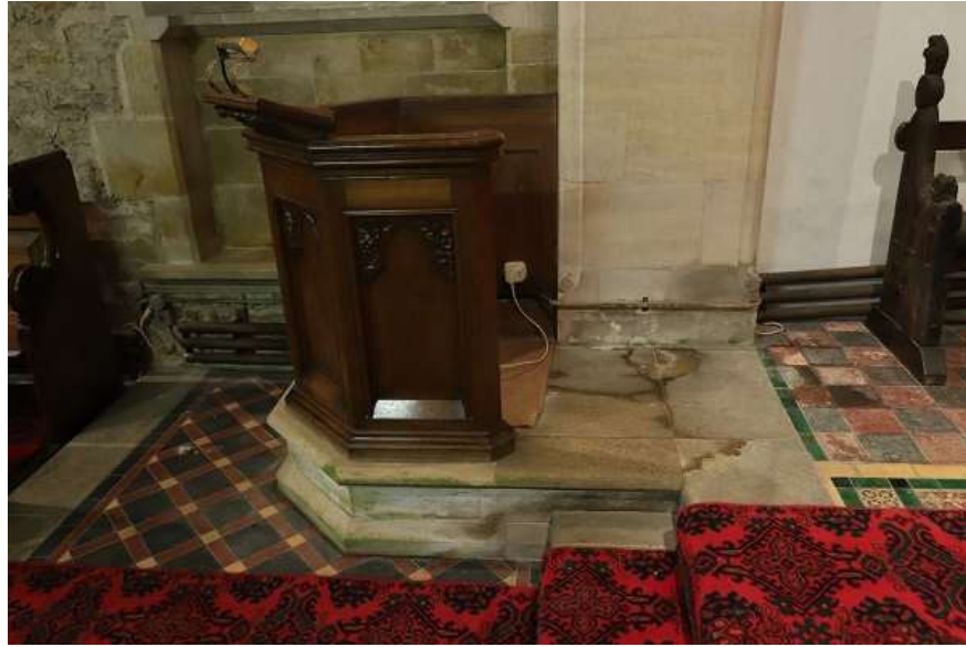
Figure 25 – Tidemarks and green mould at base of pulpit
