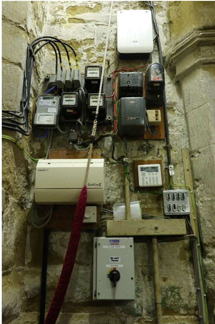
Figure 37 – Mains services in belfry
