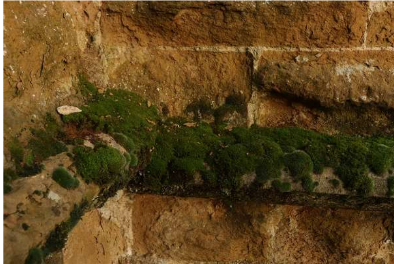
Figure 9 – Moss growth on drip course of west wall
