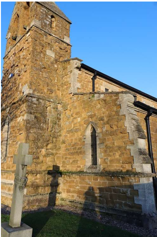
Figure 7 – Spalling to west wall
