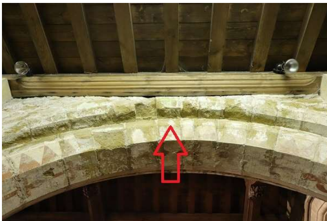
Figure 27 – Green mould growth above easternmost arch
