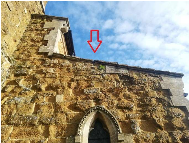
Figure 10 – Moss growth and gap in mortar of coping on west wall
