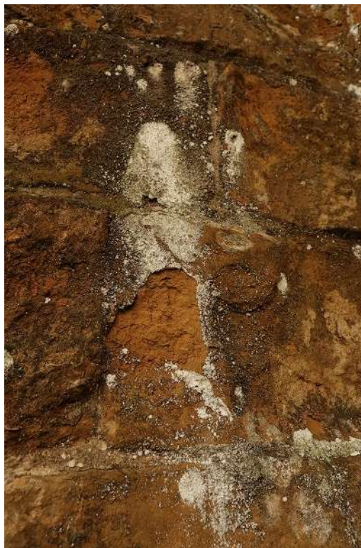
Figure 8 – Efflorescence causing spalling on north wall
