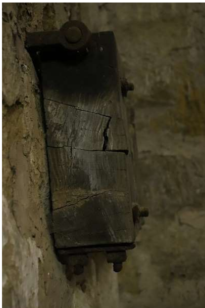
Figure 5 – Crack to wall mounted timber
