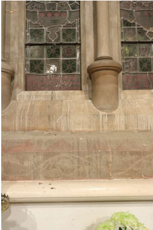
Figure 29 – Drip marks on stone and residue paint.
