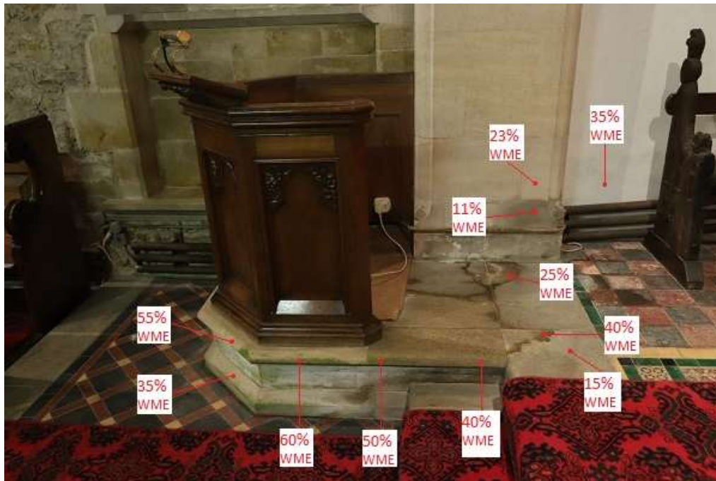
Figure 34 – GE Protimeter Mini© readings along tidemarks at base of pulpit
