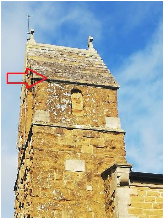
Figure 16 – Missing slate on south side of belfry roof
