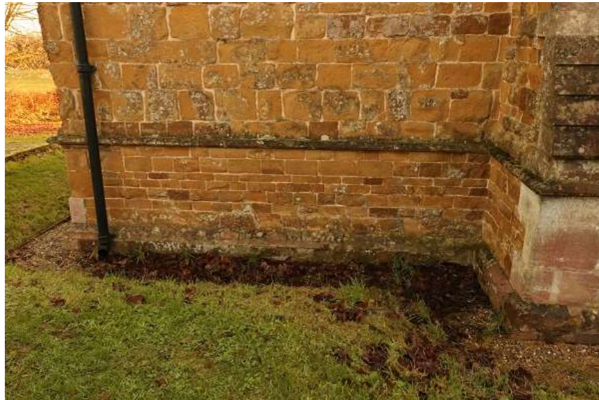
Figure 26 – Leaves blocking the french drain and gully at rear of chancel
