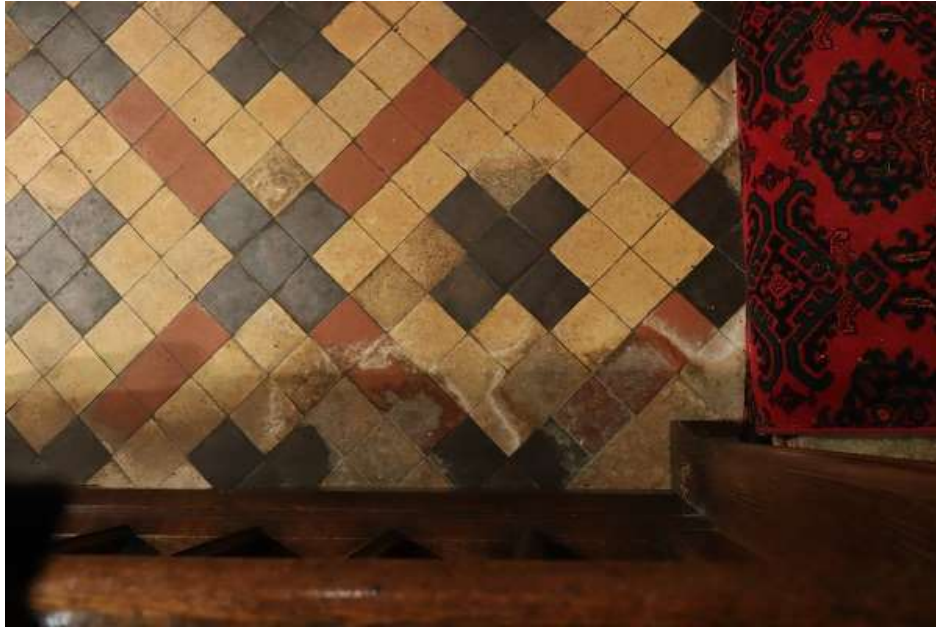
Figure 33 – Efflorescence on floor tiles
