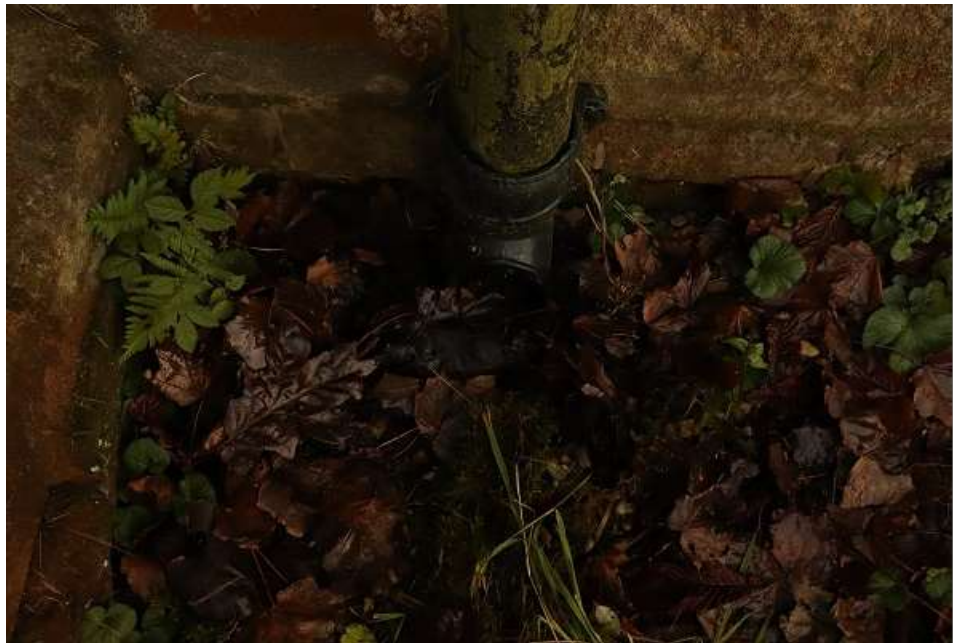
Figure 18 – Leaves and vegetation blocking drain gully
