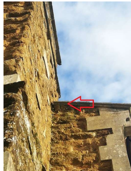
Figure 11 – Gap between coping and belfry
