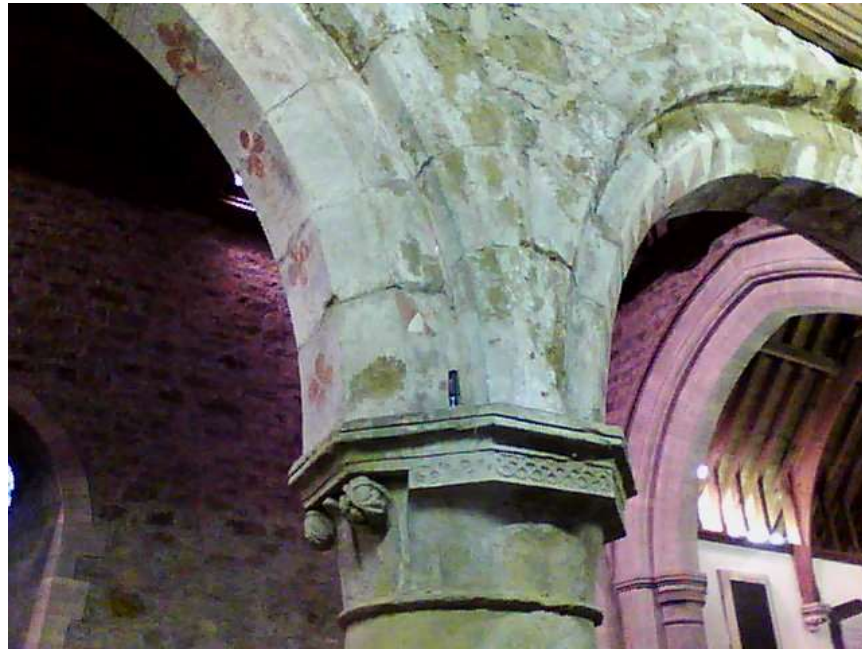
Figure 43 – Datalogger© positioned above capitol in front of painting
