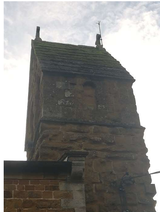
Figure 17 – Moss growth on north side of belfry roof
