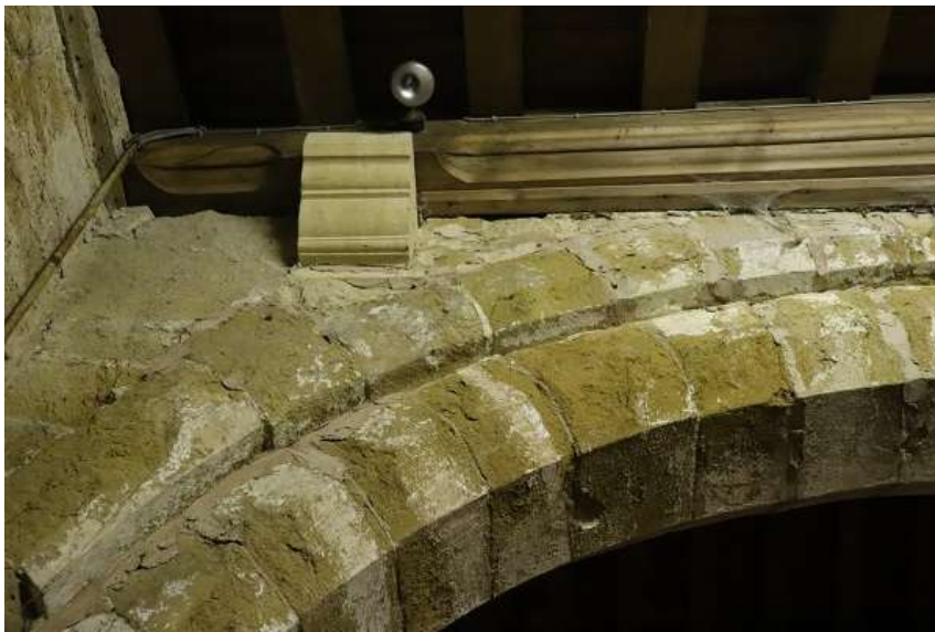
Figure 21 – Spalling of stone of west arch
