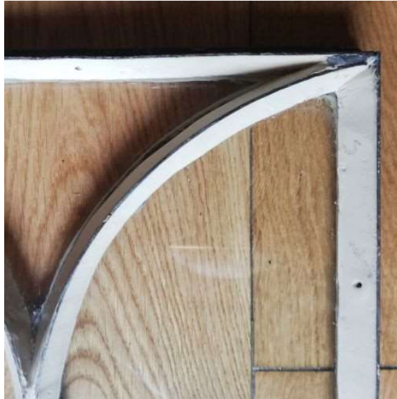
Fig.78 – Putty glazing on the interior, Casement 2
