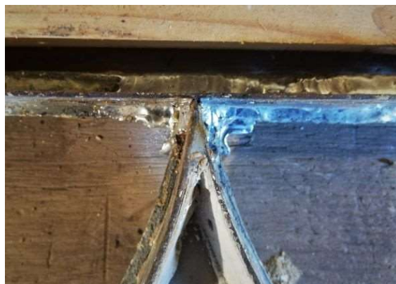
Fig.74 – New solder joint, C2
