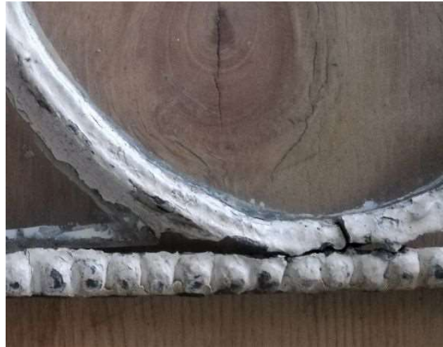
Fig.36 – Cracked joint, Casement 1.
