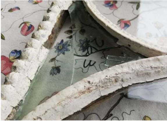
Fig.37 – Shatter pane, Casement 2
