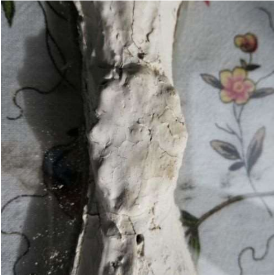
Fig.41 – Paint obscuring decorative flower, Casement 2
