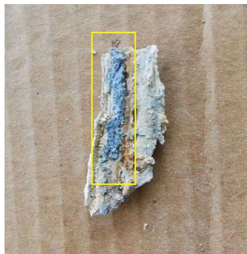
Fig.32 -Lead corrosion adhered to detached putty, C2
