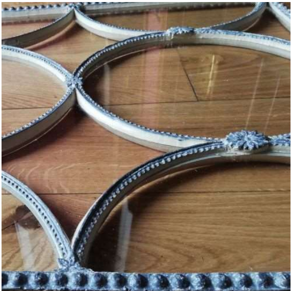
Fig.77 – Putty glazing on the front, Casement 2
