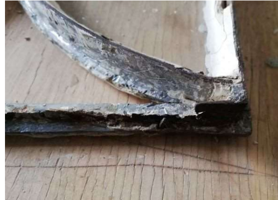
Fig.34 - Severe corrosion of bar has led to disintegration, C1
