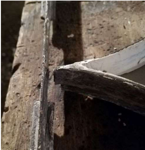
Fig.35 - Cracked and loose joints on Casement 2
