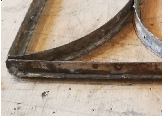
Fig.33 - Corrosion of base metal, Casement 1
