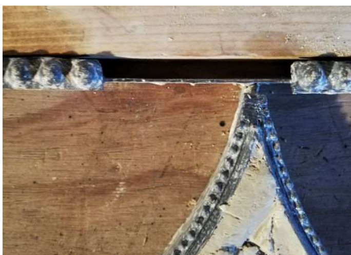
Fig.72 – Missing leadwork about loose joint, C2
