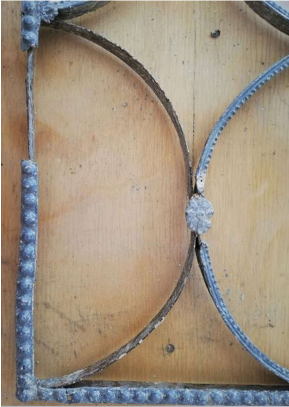
Fig.63 – Missing leadwork sections, Casement 1
