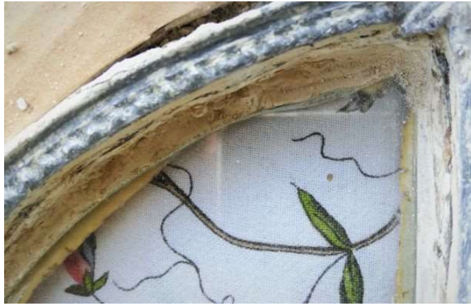
Fig. 26 – Excess putty use resulted in smaller and smaller panes, C2
