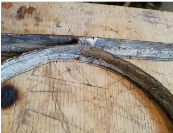
Fig.55 – Cracked solder joint and block, Casement 1
