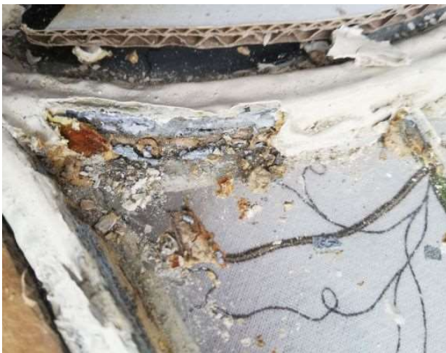
Fig.31 - Friable corroded lead discovered beneath paint, C2
