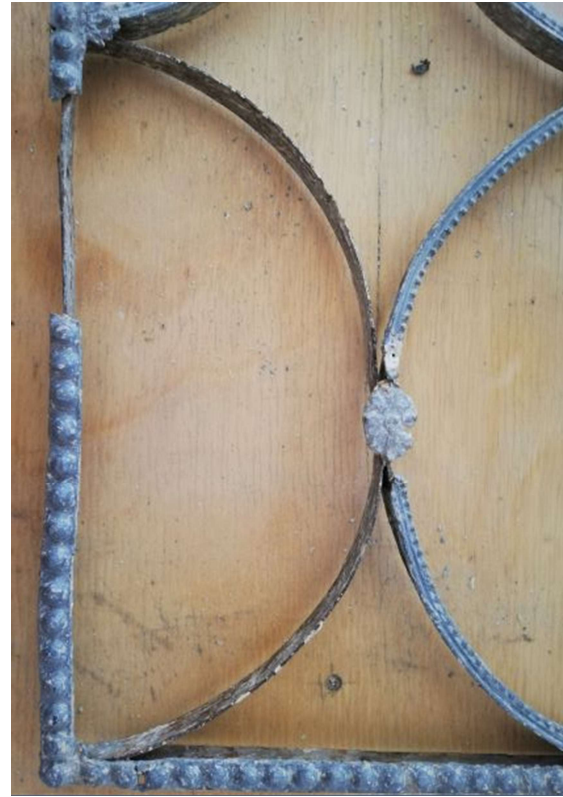
Fig.30 – Full extent of decorative lead loss evident, C1
