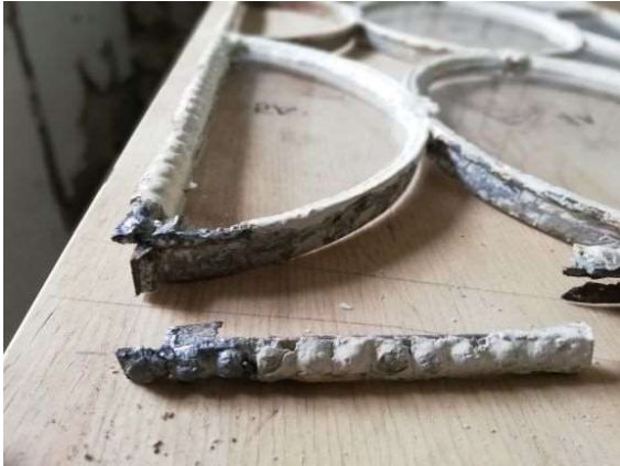
Fig.45 – Corroded flat bar and lead detached, C1
