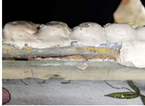
Fig.38 – Missing putty, Casement 2
