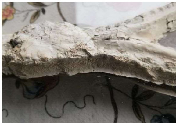
Fig.40 – Untidy application of putty, C2
