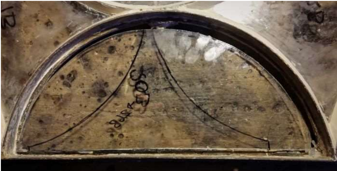
Fig.65 – Original glass that no longer fits within frame to be reused elsewhere, Casement 2
