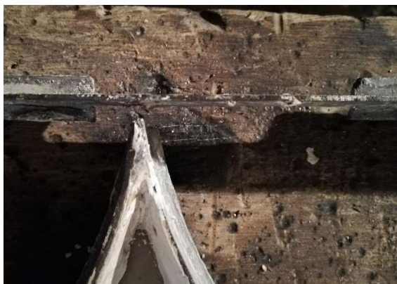
Fig.73 – Cracked and loose joint, C2
