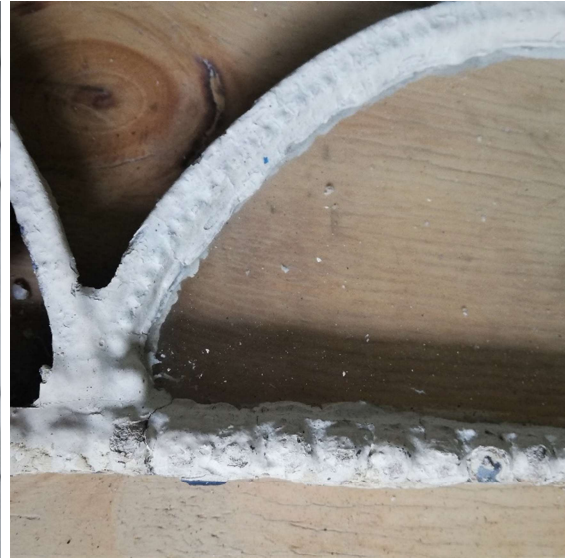
Fig.42 – Paint obscuring decorative leadwork, Casement 1
