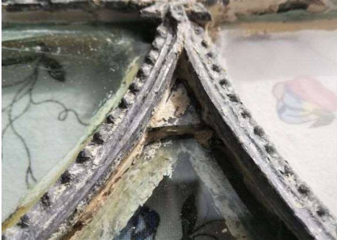
Fig.21 – Fragments of previous repairs remain in corners, C2
