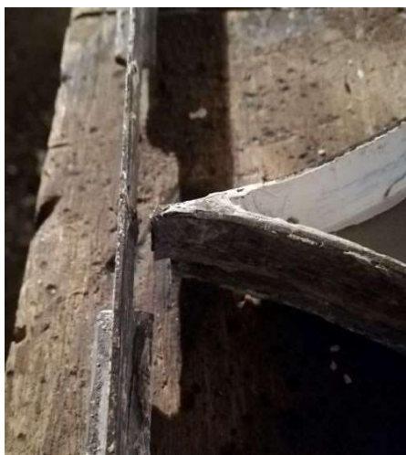
Fig.71 – Loose joint, Casement 2
